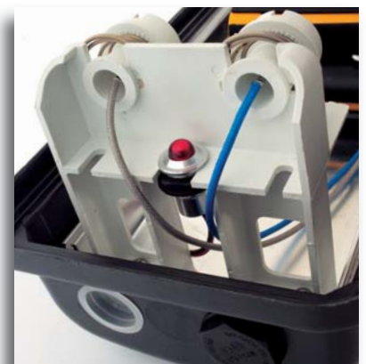
Close-up of LED battery charging light
